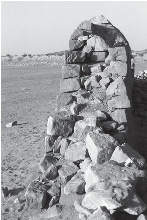
Fig. 5a: Section through wall 601/512, Building Period 6 (Hintze). Blocks of local sandstone in the shape of a truncated pyramid form the outer shell of walls. The core of the wall consists of sandstone rubble and earth mortar. No coat of plaster.
